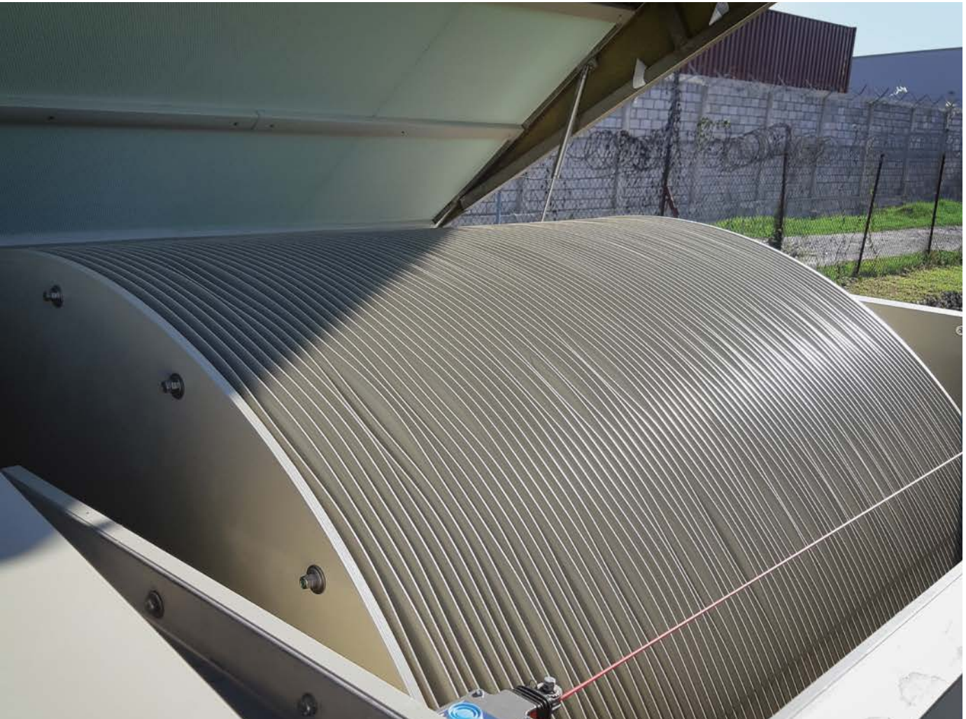
The system, based on an Ecodisk® biodisk, was installed by Veoliaforce volunteers at a hospital managed by MSF in Haiti.
